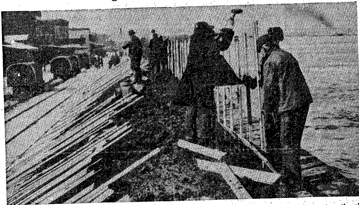
Workmen are pictured building up the Mississippi river levees at Cairo, Ill., in an effort to stem the rising waters. The most disastrous flood in the history of the father of waters cost hundreds of lives, rendered more than a million people homeless and caused hundreds of dollars worth of damage.
