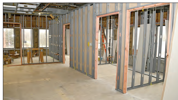
The pain clinic, being moved from its basement space to the third floor, is a completely new build out.
