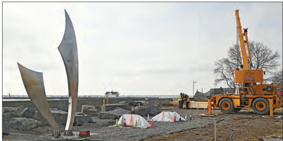
Below, two pieces of the left structure, “The Wings of Hope,” are the first to be installed March 1, as 13 more wait in nearby crates.
