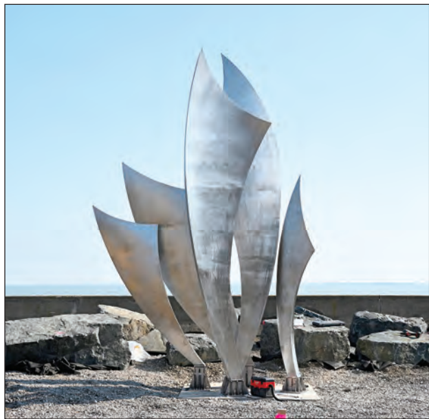
Installation of the left portion of the monument, “The Wings of Hope,” completed Wednesday. Each of the three sections will incorporate five stainless steel pieces.
