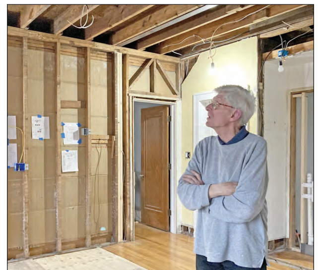
Fred Rottach, 72, helped a construction crew install steel support beams during the renovation of his house.
