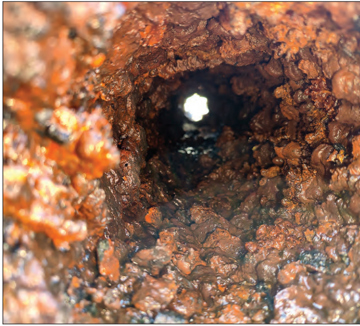
Tuberculation is the fancy name for rust inside cast iron water pipes, a section of which is shown. It is harmless, a natural condition of old cast iron and restricts the flow of water through pipes, all of which is avoided by installing pipes made of plastic.
