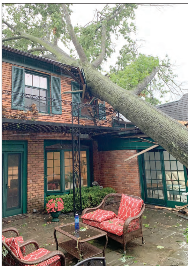
The Boggs family rushed to the basement just as this 15,000-pound oak came crashing into the second-floor bathroom of their Tonnacour home.
