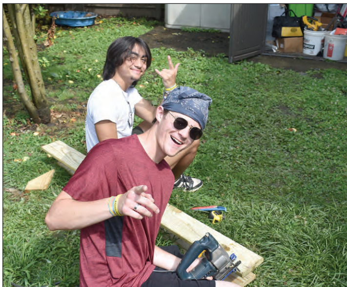
Left, Jack Bidigare, a 2023 graduate of Grosse Pointe North High School, builds a deck with a new friend made at Workcamp.
