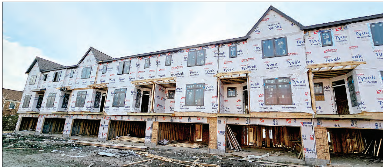
The back of the townhomes, facing the former school administration building, feature a two-car garage and small, second-floor balcony.
