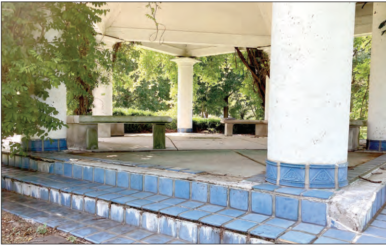
Cracked and missing Pewabic tiles typify broken steps at the Patterson Park gazebo.
