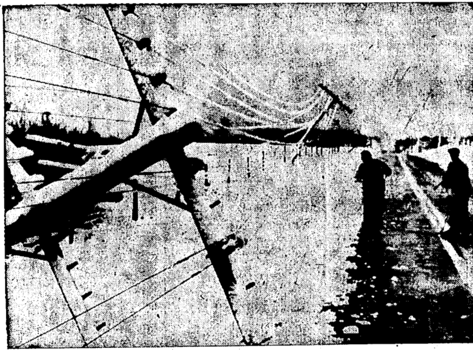
OUT OF ORDER—Telephone linemen begin the chill job of repairing those snow-downed lines south of Crandon, Wis., where an introductory 10 inches of wet snow wrought havoc.
