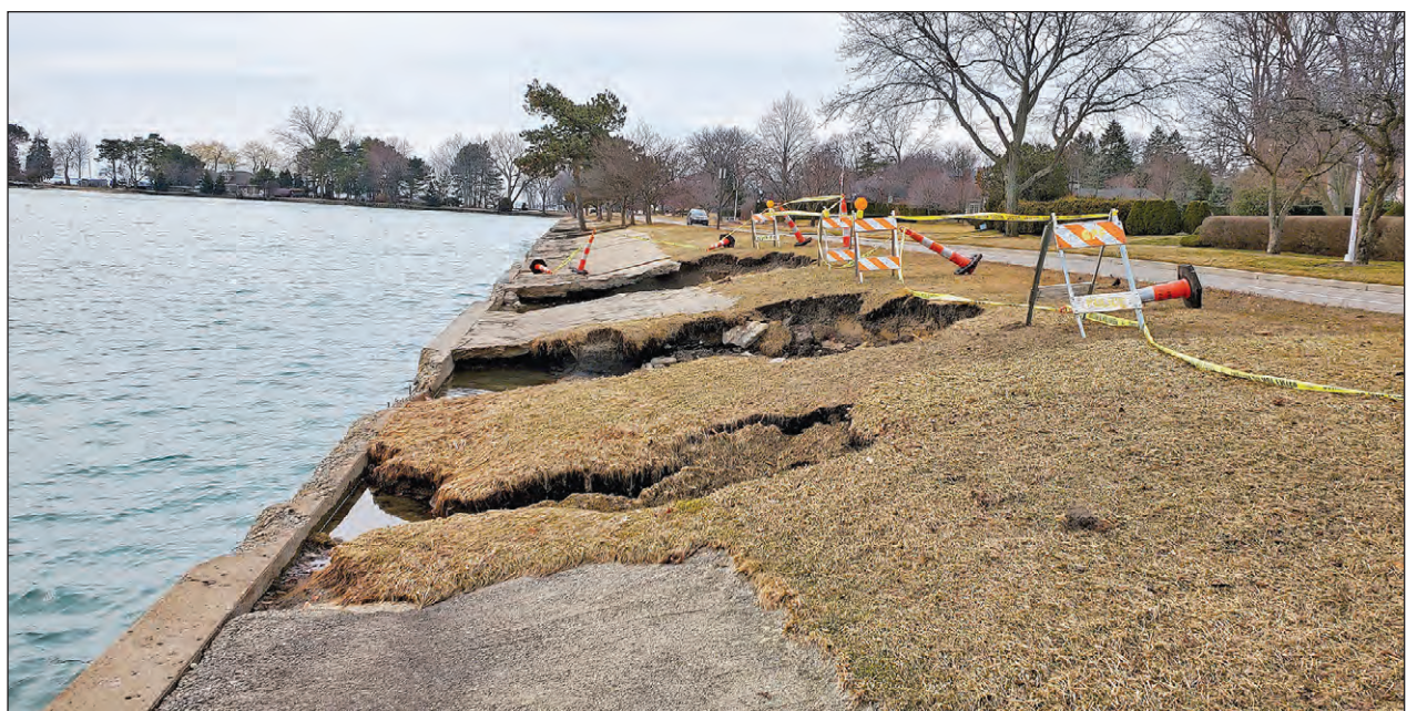
Grosse Pointe Farms took steps to address sinkholes along the seawall in March.
