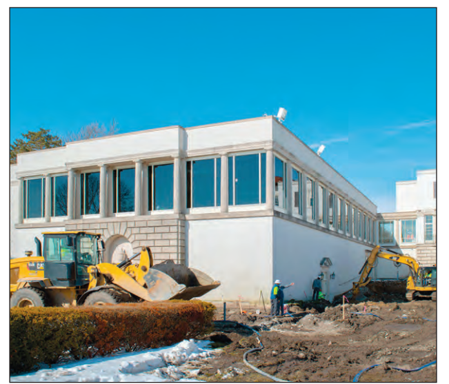
Physical site work has begun, including prepping the foundation of The War Memorial ballroom to create a watertight space along the lakeside of the building.
