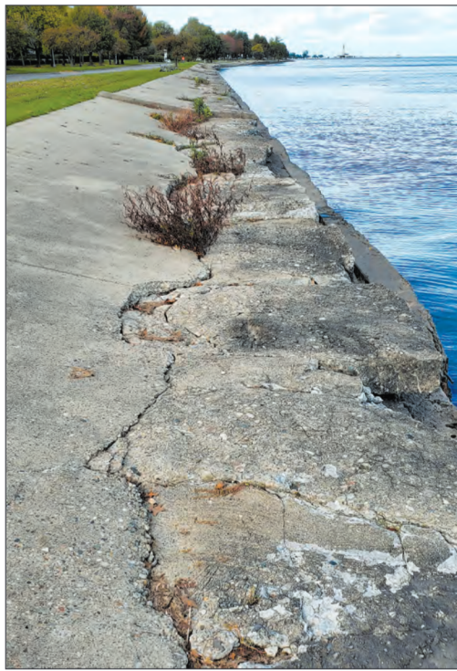
PHOTO BY RENEE LANDUYT Construction of a new seawall along the three-mile stretch of Lakeshore is estimated to cost $25 million to $30 million.
