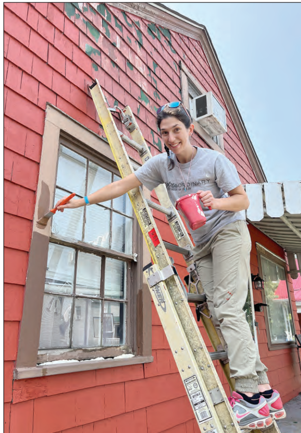
Renata Conger got to work adding a fresh coat to a house in need of a paint job.
