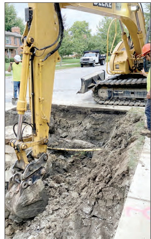
Under guidance from a crew mate, the operator of an excavator carefully positions the boom between a water line, at lower left, a man-hole opening and another underground utility line.
