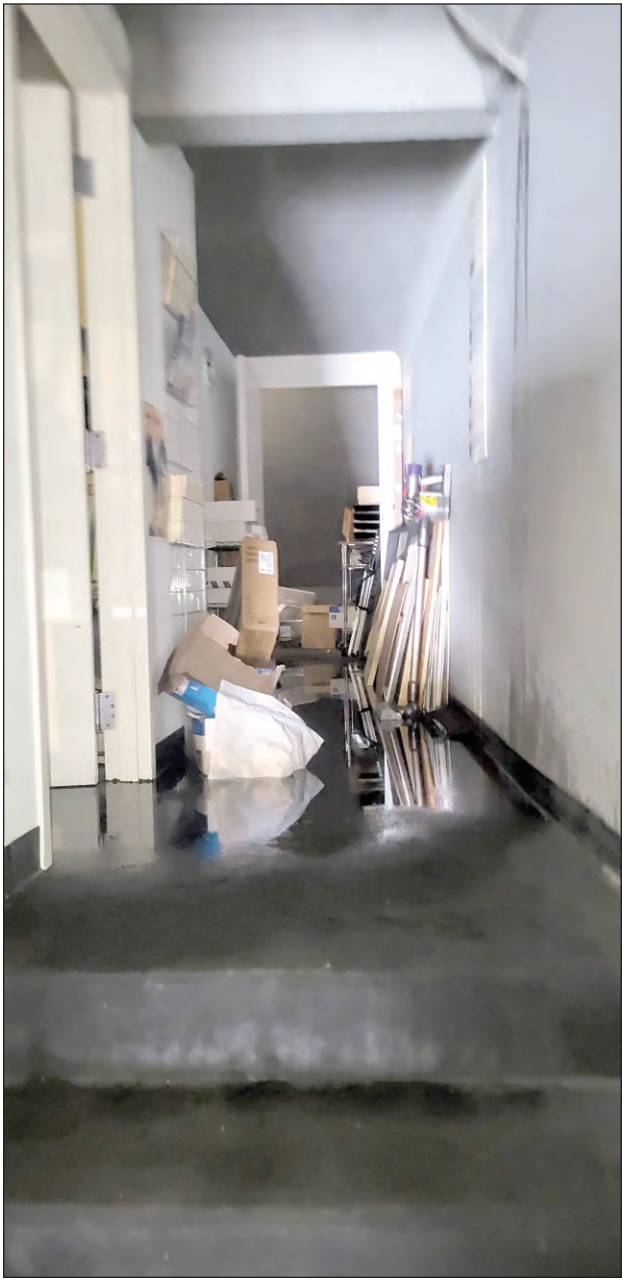
Floors throughout DAM were saturated following the flood.
