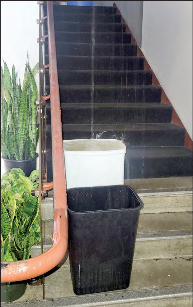
A stream of leaking water overflows from one garbage can into another after on the DAM staircase.
