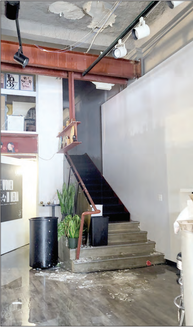
Chunks of plaster lay on the main floor of DAM after water compromised the ceiling.
