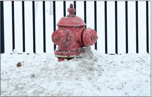
Left, a hydrant along Grosse Pointe Boulevard, near The Grosse Pointe Academy, that needs to be cleared. Right, a hydrant along Grosse Pointe Boulevard, down the street from The Grosse Pointe Academy, that is cleared of snow.
