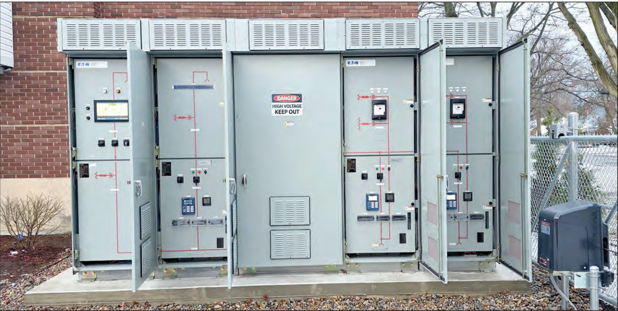
A look inside the switching gears that operate the generator.
